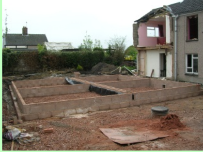
After demolishing the extension and clearing the ground, the builders laid foundations and started to build the walls.
