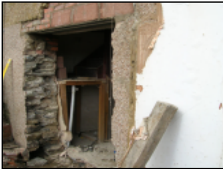
Above: hole in back wall at Broadwell
